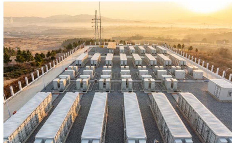
Power play Battery storage is in demand
